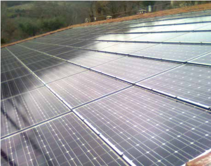
Solrif-framed 20 kWp installation on residential rooftop in Italy
